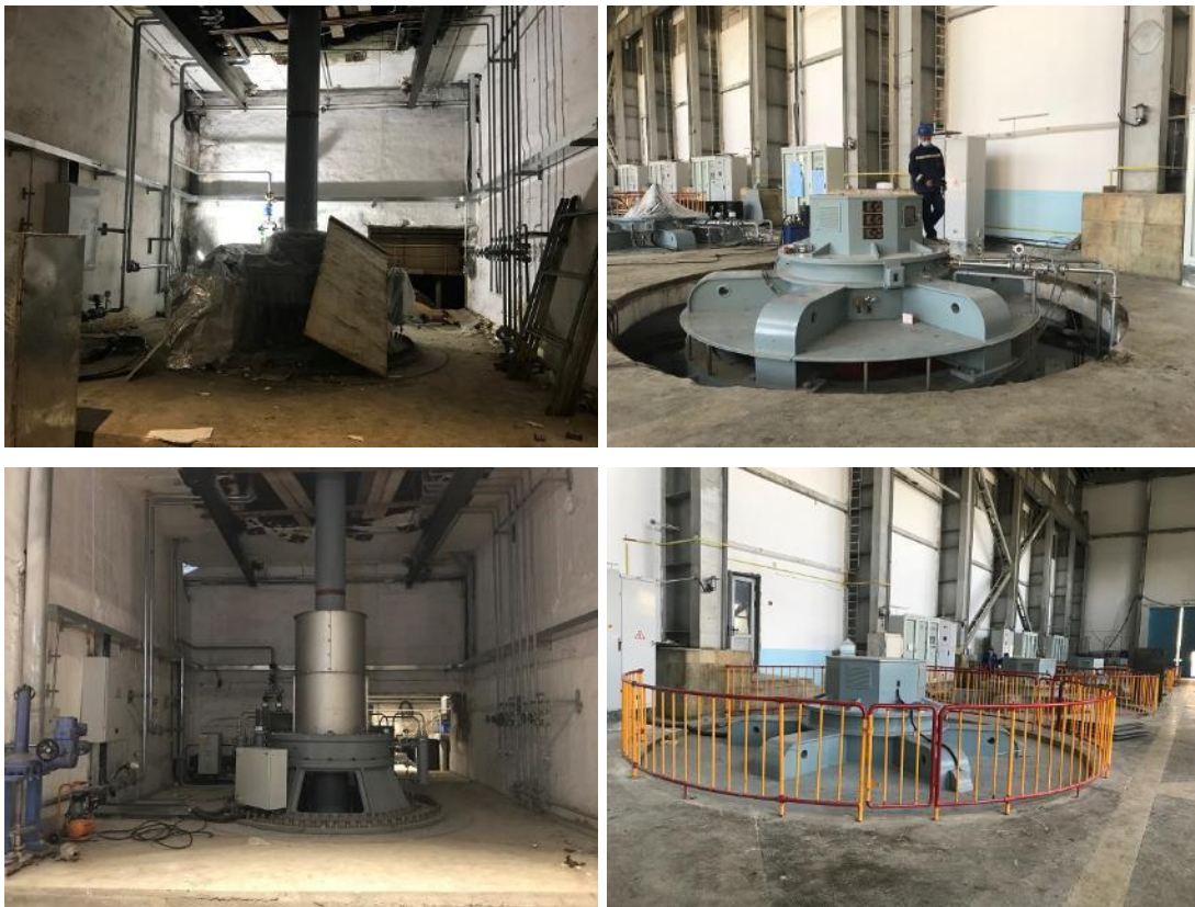
Installation Works of the Pump Units #6 and 7 in Kizil Tapa Pump Station (ABISRP 03 Lot 2)
