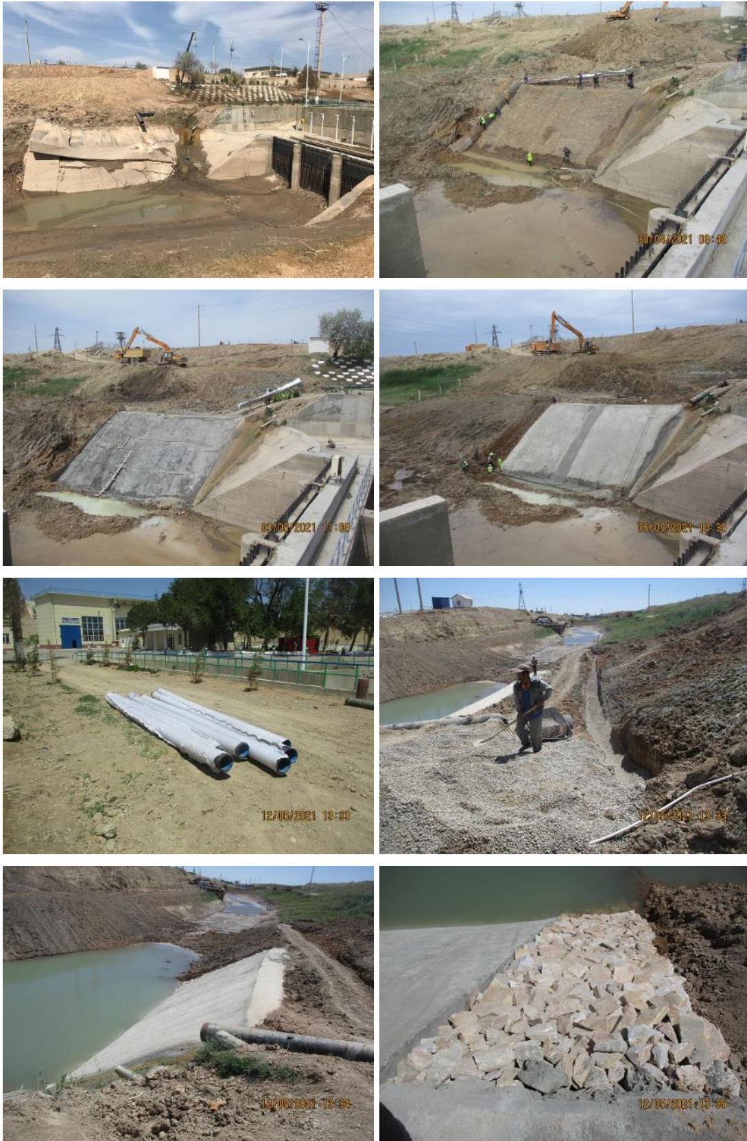
Reconstruction of Damaged Slope Protection Concrete at the Upstream of Trashrack Structure on Canal KM of Kuyu Mazar Pump Station (ABISRP 03 Lot 1)
