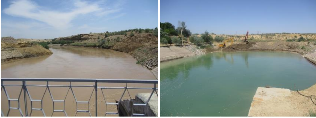
Removal of Cofferdams upon Completion of Rehabilitation Works on Regulator ABMK-2 at Hydrosystem Prokop (ABISRP 02)
