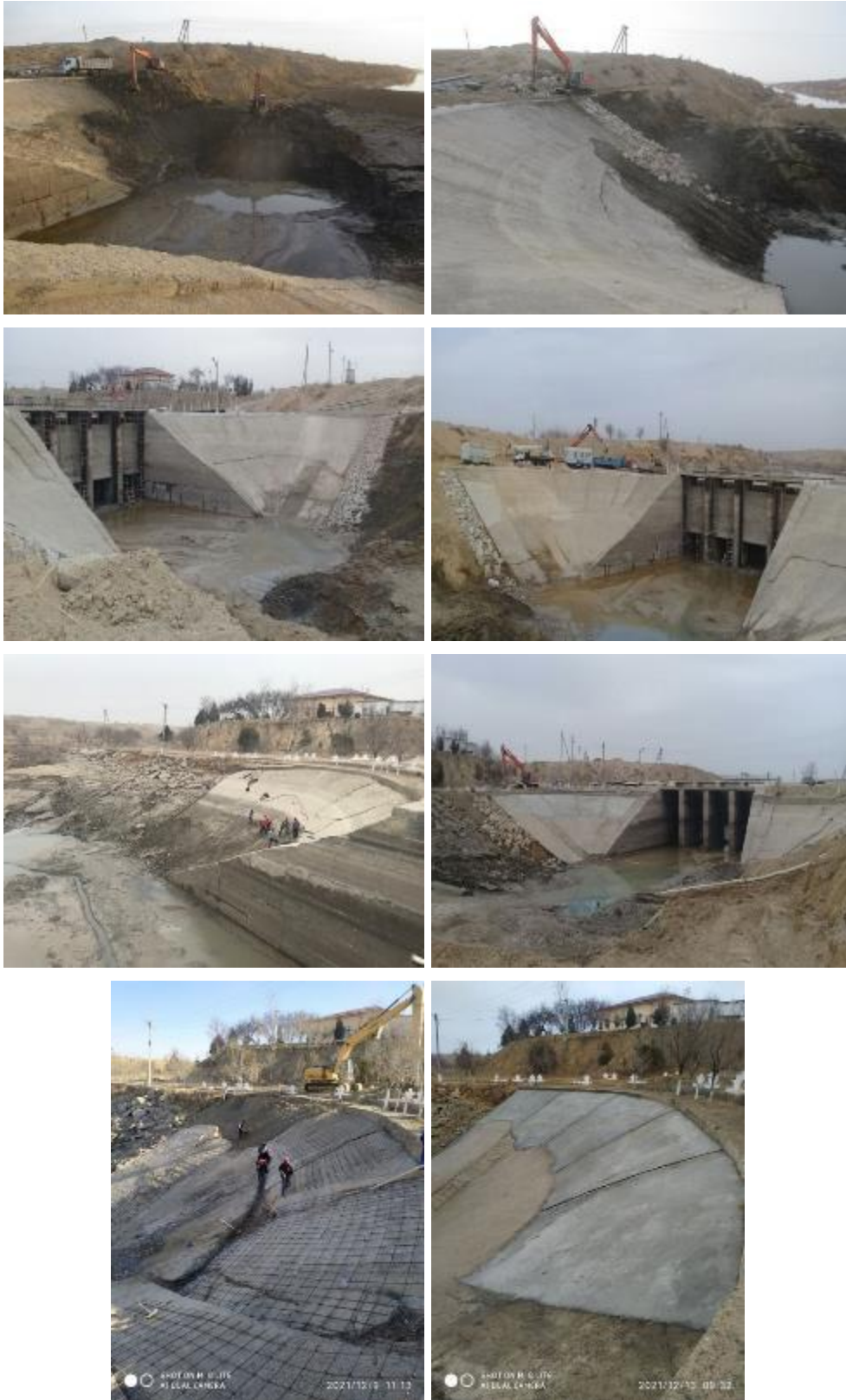
Photos above are from December 2021 Rehabilitation of Slopes on Outflow-Tudakul at Hydrosystem Prokop (ABISRP 02)
