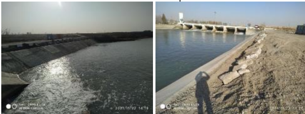
Photos above are from November 2021 Slope Concrete Reconstruction Works at the Downstream of Regulator Zarafshan at Hydrosystem Tashrabad (ABISRP 02)
