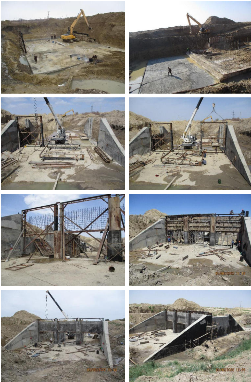
Construction of the Bypass Structure ABK-1 at Hydrosystem Troynik (ABISRP 02) All photos are taken in the months of May, June 2022
