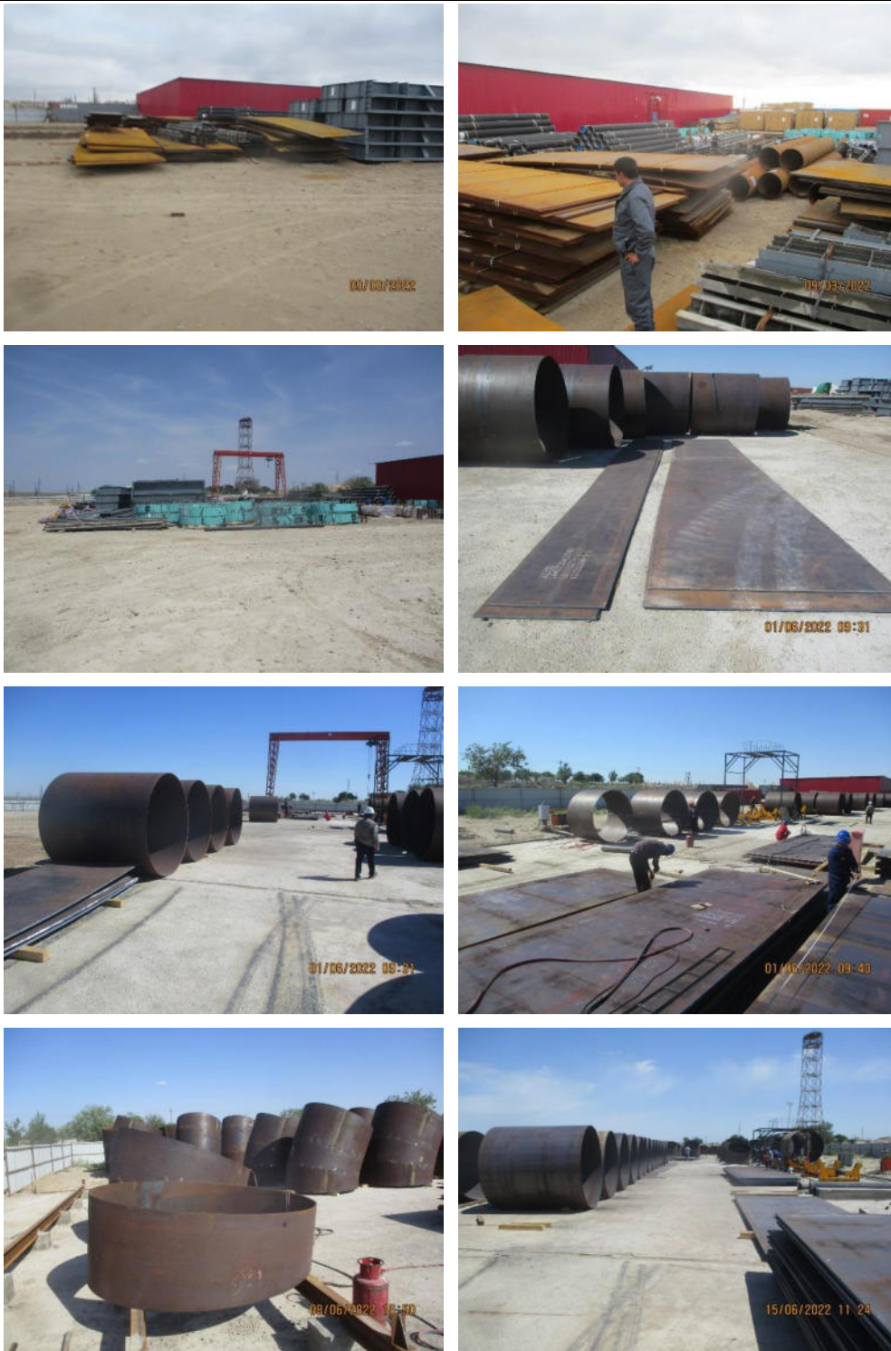
Manufacturing of Discharge Pipes at the Workshop at Site (ABISRP 01) All photos are taken in the months of March, June 2022
