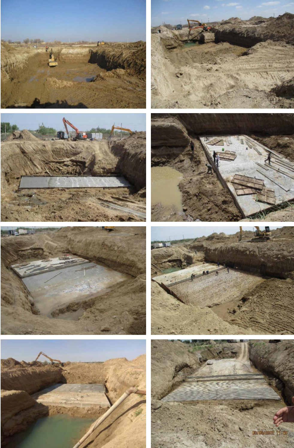
Construction of the Bypass Structure ABK-2 at Hydrosystem Troynik (ABISRP 02) All photos are taken in the months of May, June 2022
