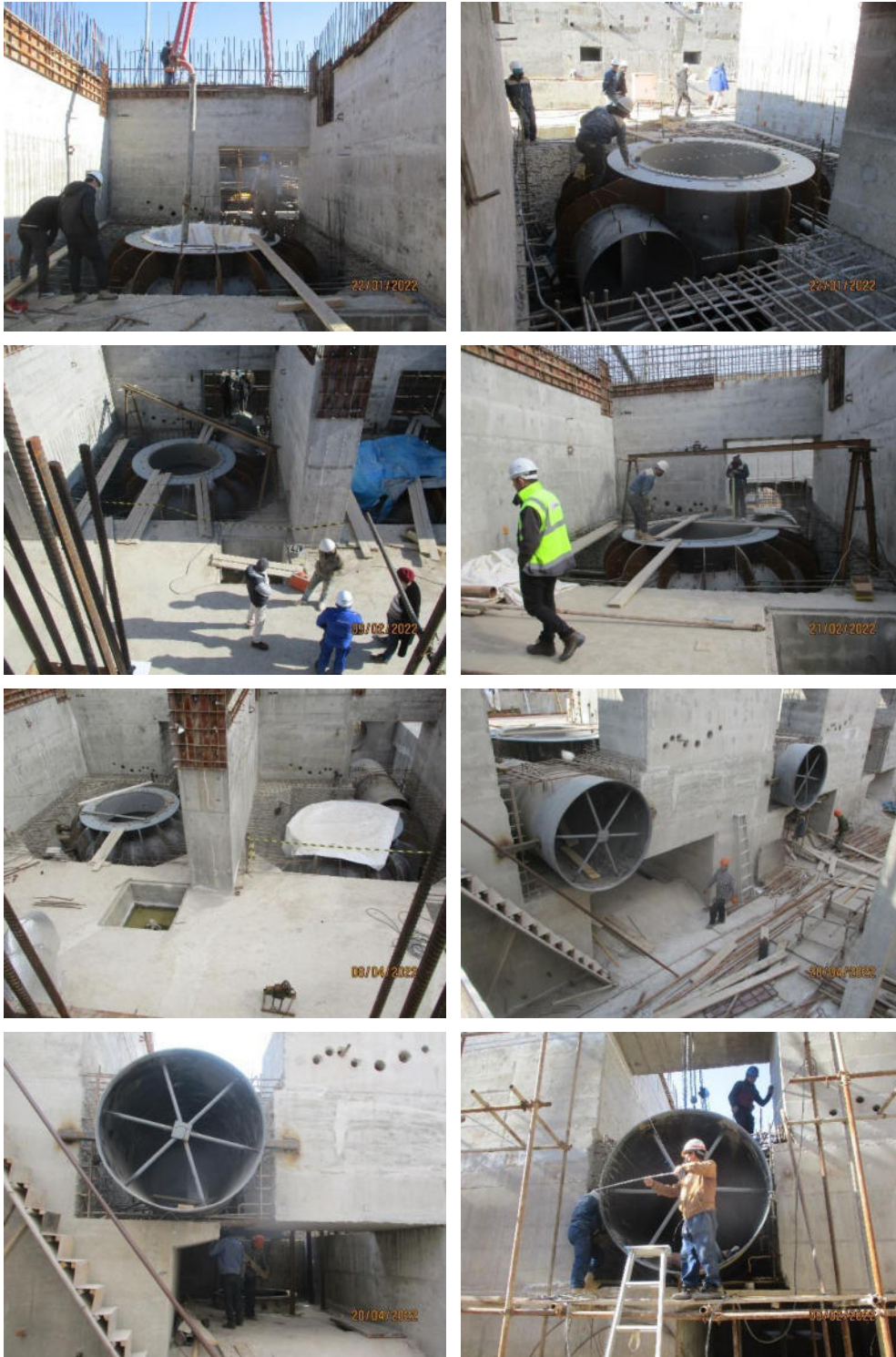
Installation Works of the Volute (Spiral) Casings of the Main Pumps (ABISRP 01)
