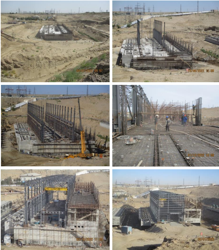
Construction Works of the Aboveground Part (Superstructure) of the Pump Station Building (ABISRP 01)
