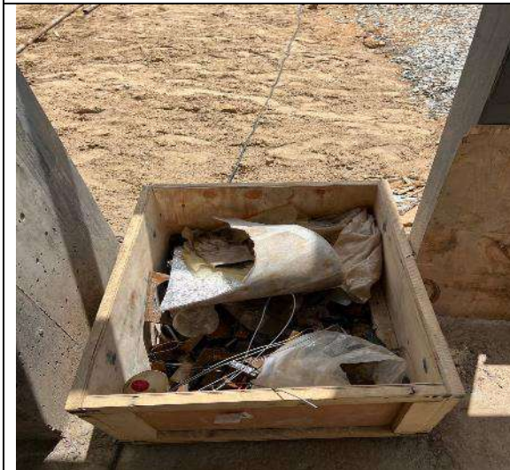
3. Construction materials and other wastes not segregated.
