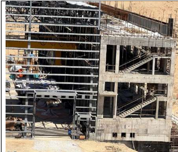
1. Construction of pumping station. Working at height without safety signs and instruction/boards.
