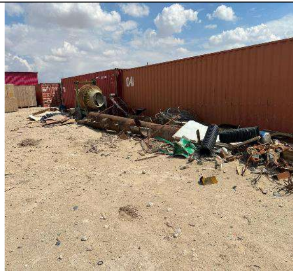
4. Different kind of wastes and construction materials not segregated.
