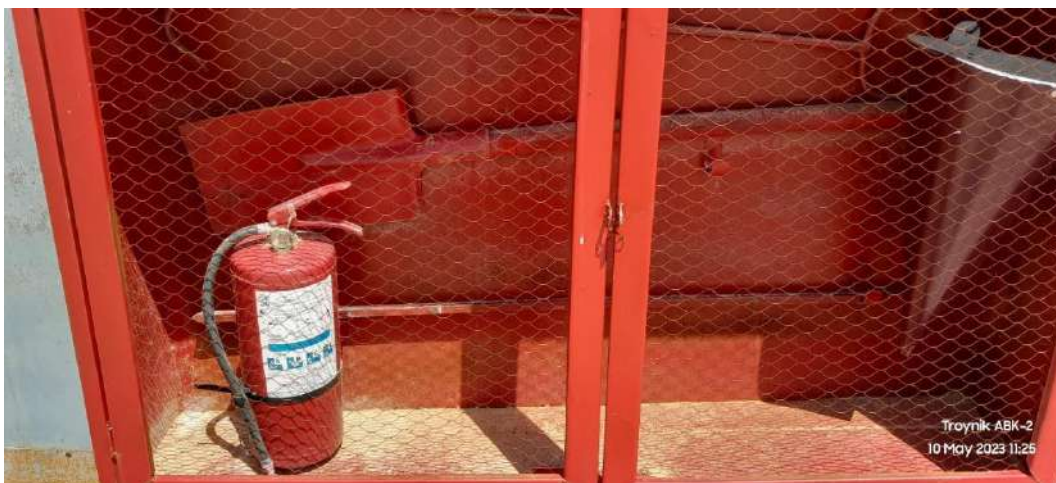
Photo 2: Locked fire cabinet
